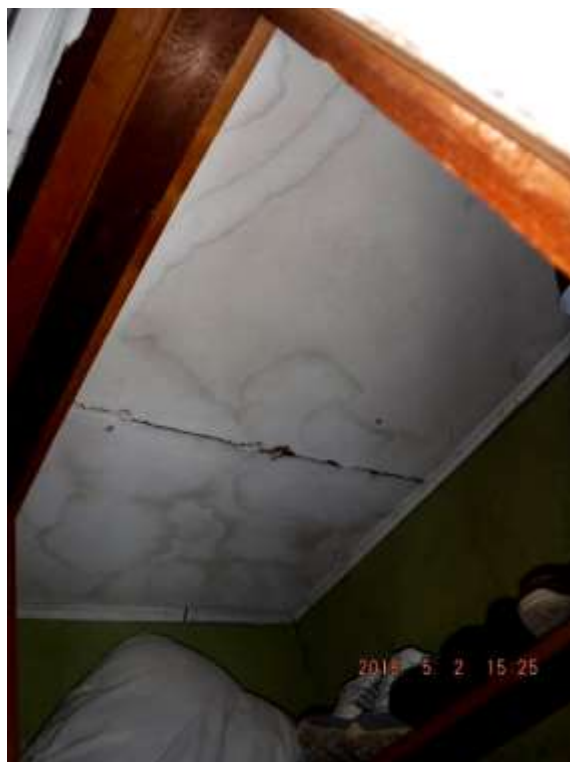
Figure 15 Water stains on closet; see roofing section comments.
