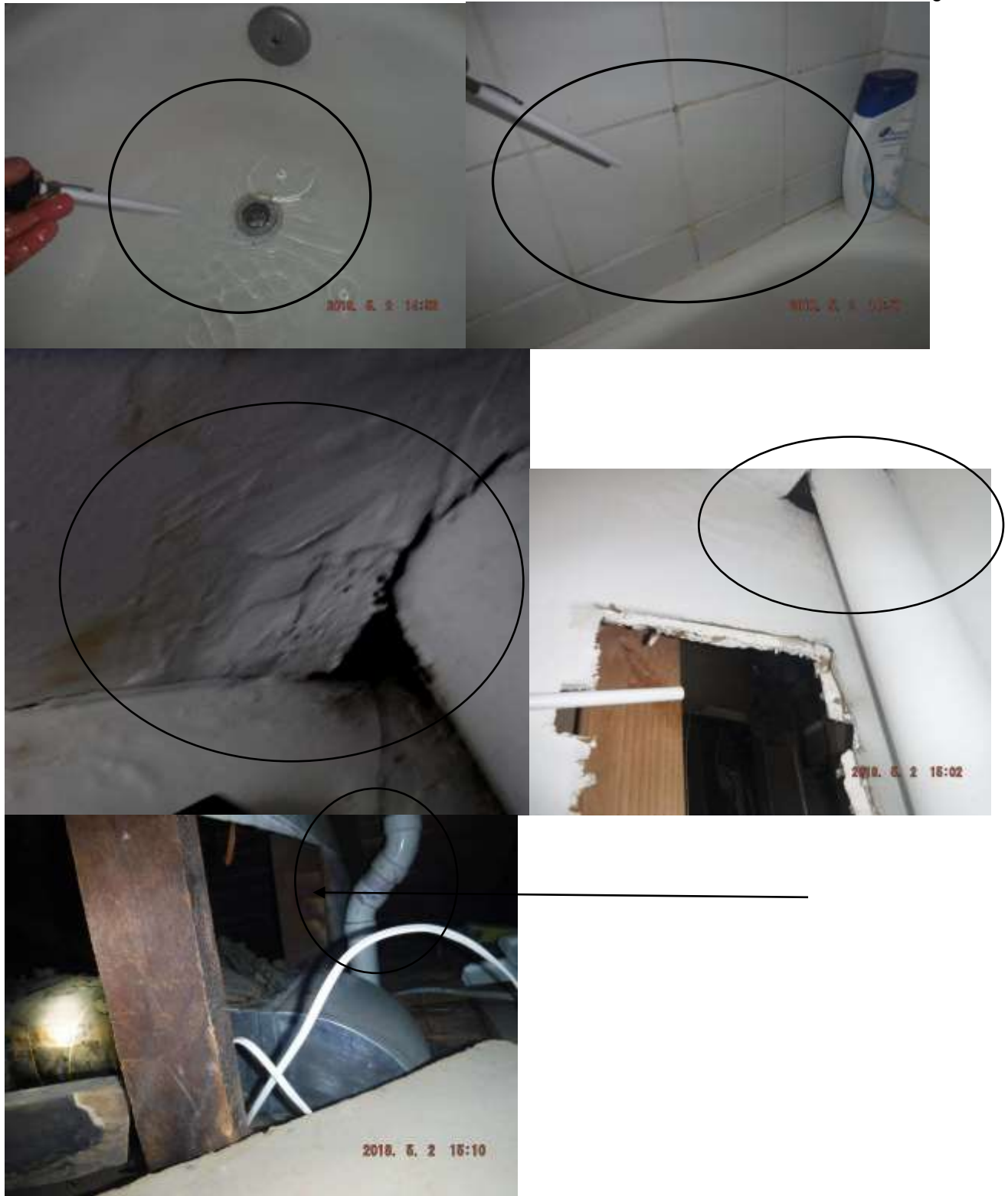
Figure 13 There was yellowing/water stains around a plumbing vent. See roofing section comments.
