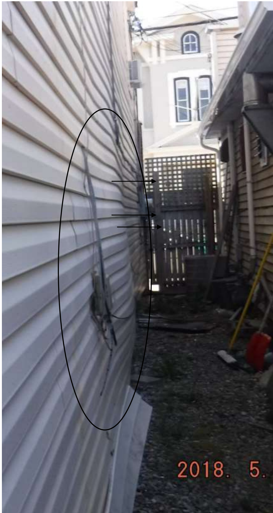
Figure 7 Example of bulging walls; left side depicted. There were bulges on left and right as well as upper and lower. There were structural concerns in the home ( flooring, roof, etc.).
