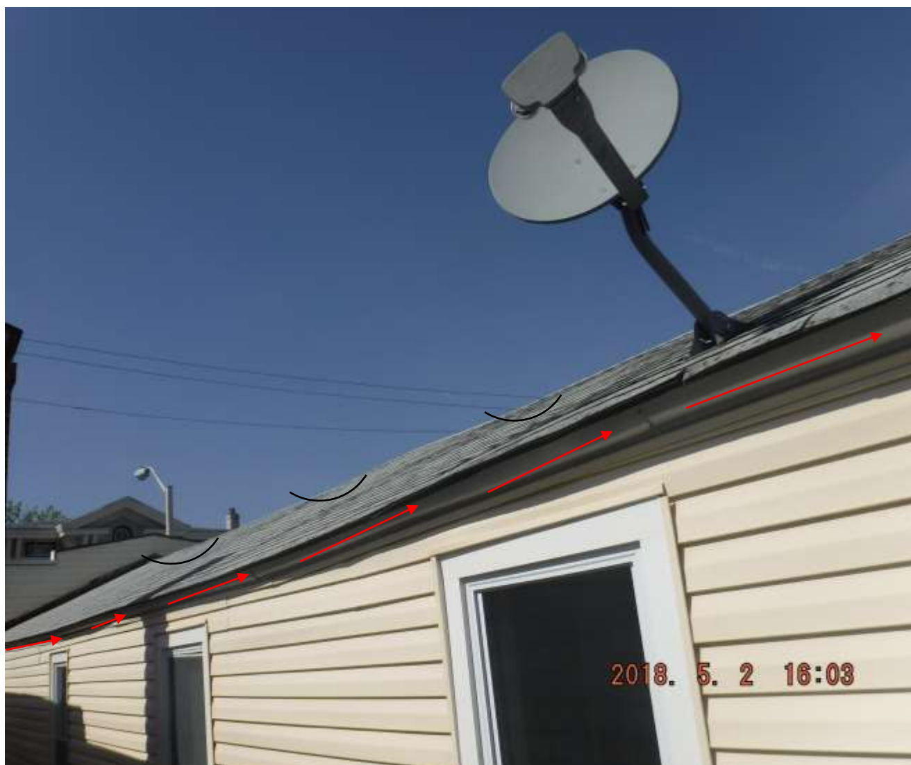
Figure 6 Walls on both sides were bowed and roof had waviness, depressions and structural deficiencies. Recommend further evaluation by a structural engineer (PE), roofer and or building contractor along with the structure of the building. See siding section comments.
