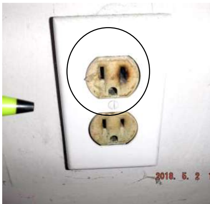
Figure 12 Recommend a licensed electrician evaluate scorched outlet and make repairs/replacement; overloaded or heavy draw appliance. Discuss all electrical needs with the electrician for the apartment and the business needs and upgrade and install power, devices, outlets, fixtures, lighting, etc.
