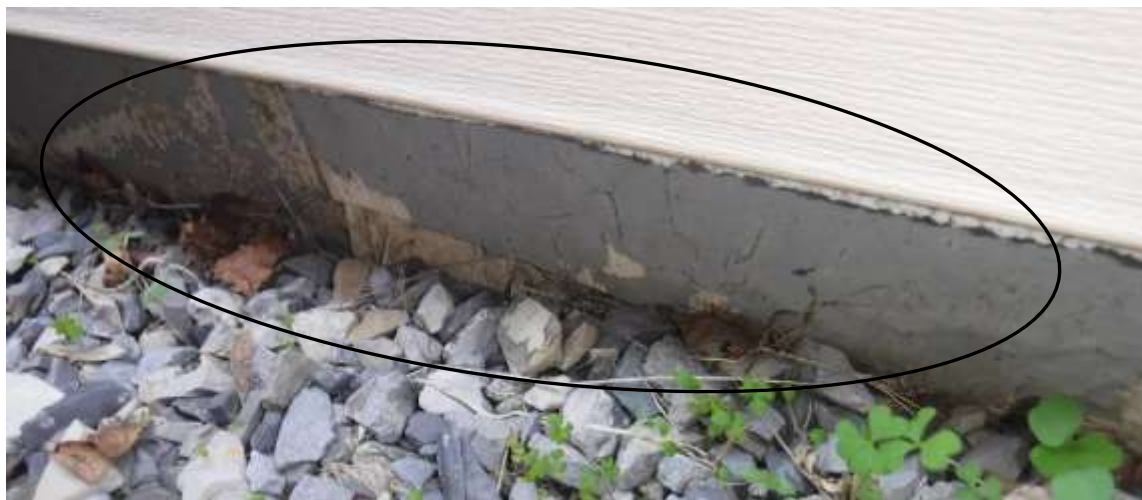
Figure 8 Visible asbestos like siding (painted gray) slipped down and loose under the vinyl siding.
