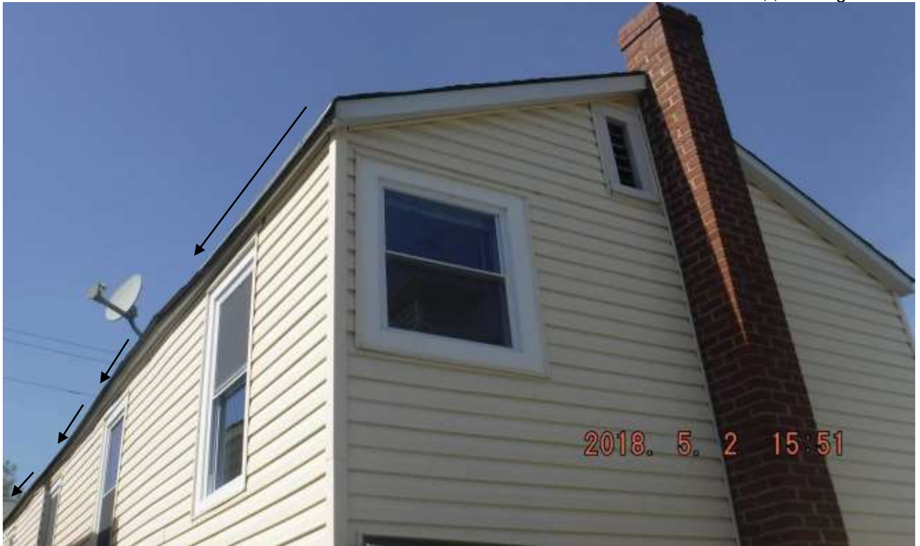
Figure 5 Asphalt tab roof over cedar shingles (no sheathing), past life, no gutters, poor ventilation & insulation and structural concerns/deficiencies.
