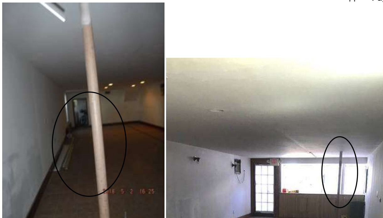
Figure 11 Two visible lally columns and structural concerns in the building. Follow up with the structural engineer (PE) for evaluations before closing & contractual limitations.
